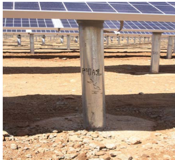
Figure 1. Typical solar array installation showing land grading and vegetation removal. Photo by Brenda Beatty, NREL
